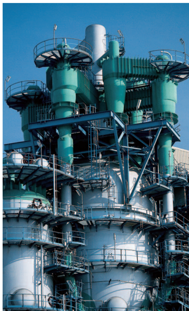
The residue catalytic cracker complex at SRC
