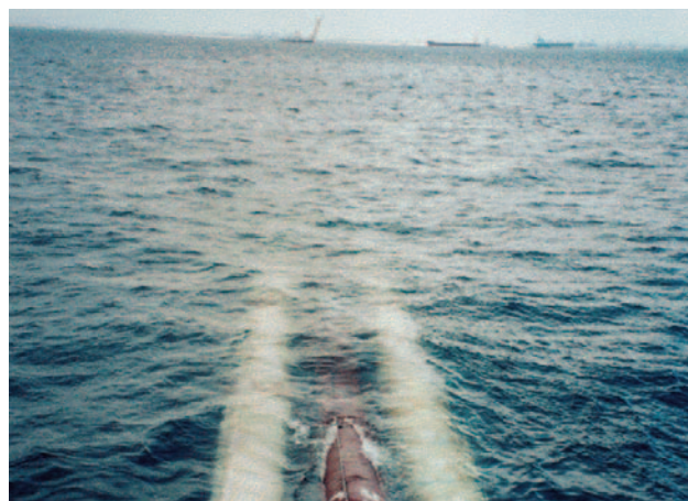
The Grissik-Batam-Singapore Pipeline was commissioned on 4 August 2003
